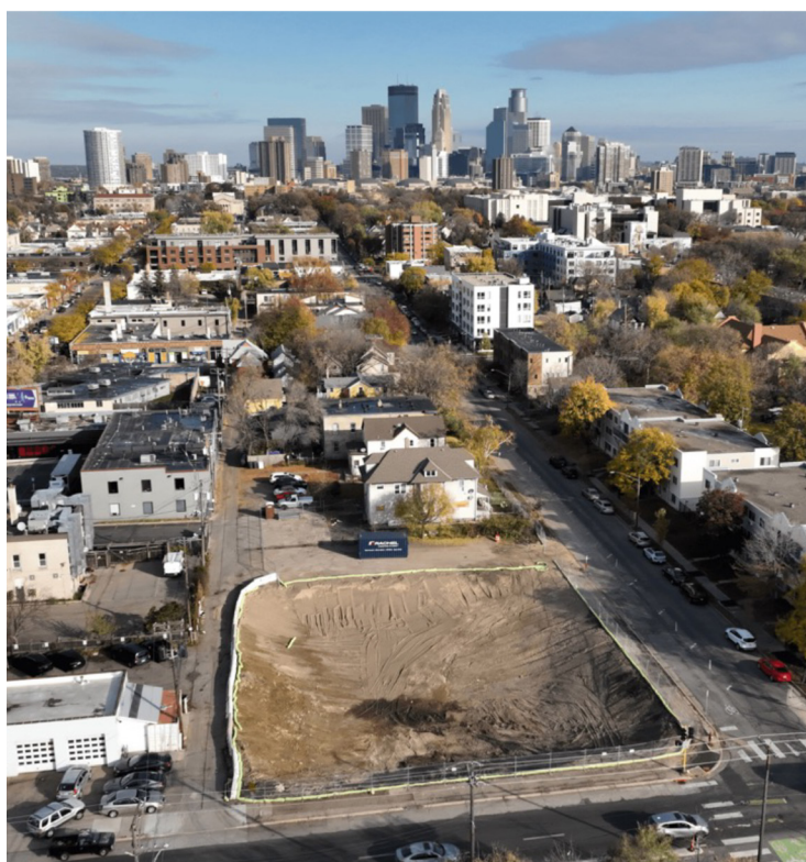
On Wednesday, June 12, 2024, Simpson House broke ground on the construction of their new facility!
